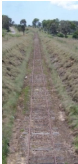
Part of Australia's future? The Main North Line at Tenterfield heads for Queensland.
