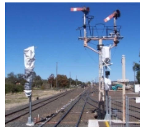
Last days of the semaphore signals at Werris Creek, 11th August, 2007, with the new electric signals controlled from Broadmeadow waiting to be unveiled.
